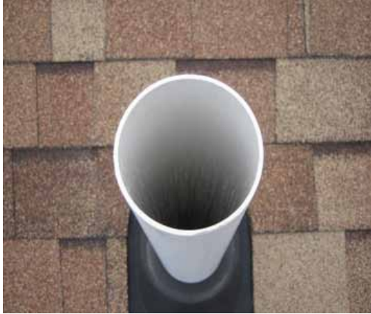
Figure 13. Example of Radon Pipe End with No Screen
