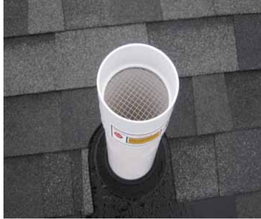
Figure 14. Example of Radon Pipe End with Screen
