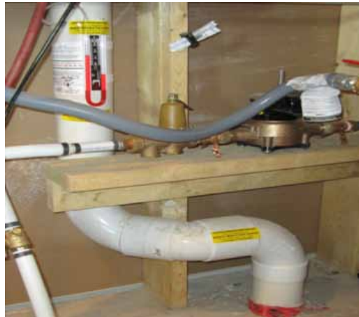
Figure 2. Example of Pipe Labeled
