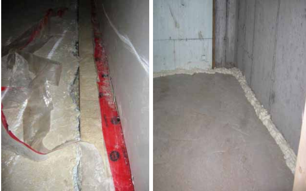
Figure 9. Example of Inadequate Sealing of Slab Edges Figure 10. Example of Slab Edges Sealed with Spray Foam
