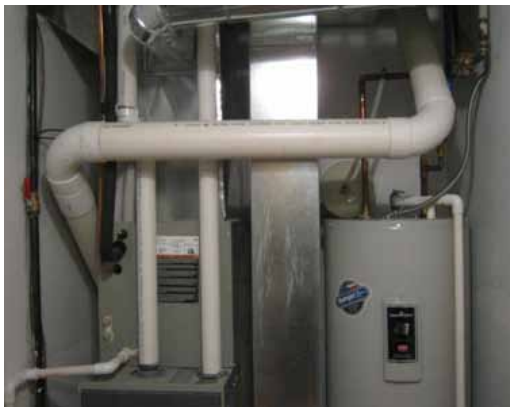
Figure 7. Example of Pipe Run Unsupported
