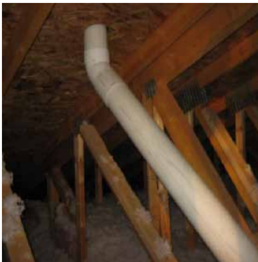
Figure 15. Example of Passive Pipe with No Electrical Provisions
