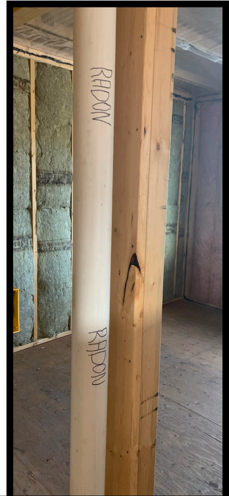
Figure 11: Radon labelling on a vent pipe. The informal and non-standardized labelling is typical. Photo credit: Chantal Wilson as part of this study.
