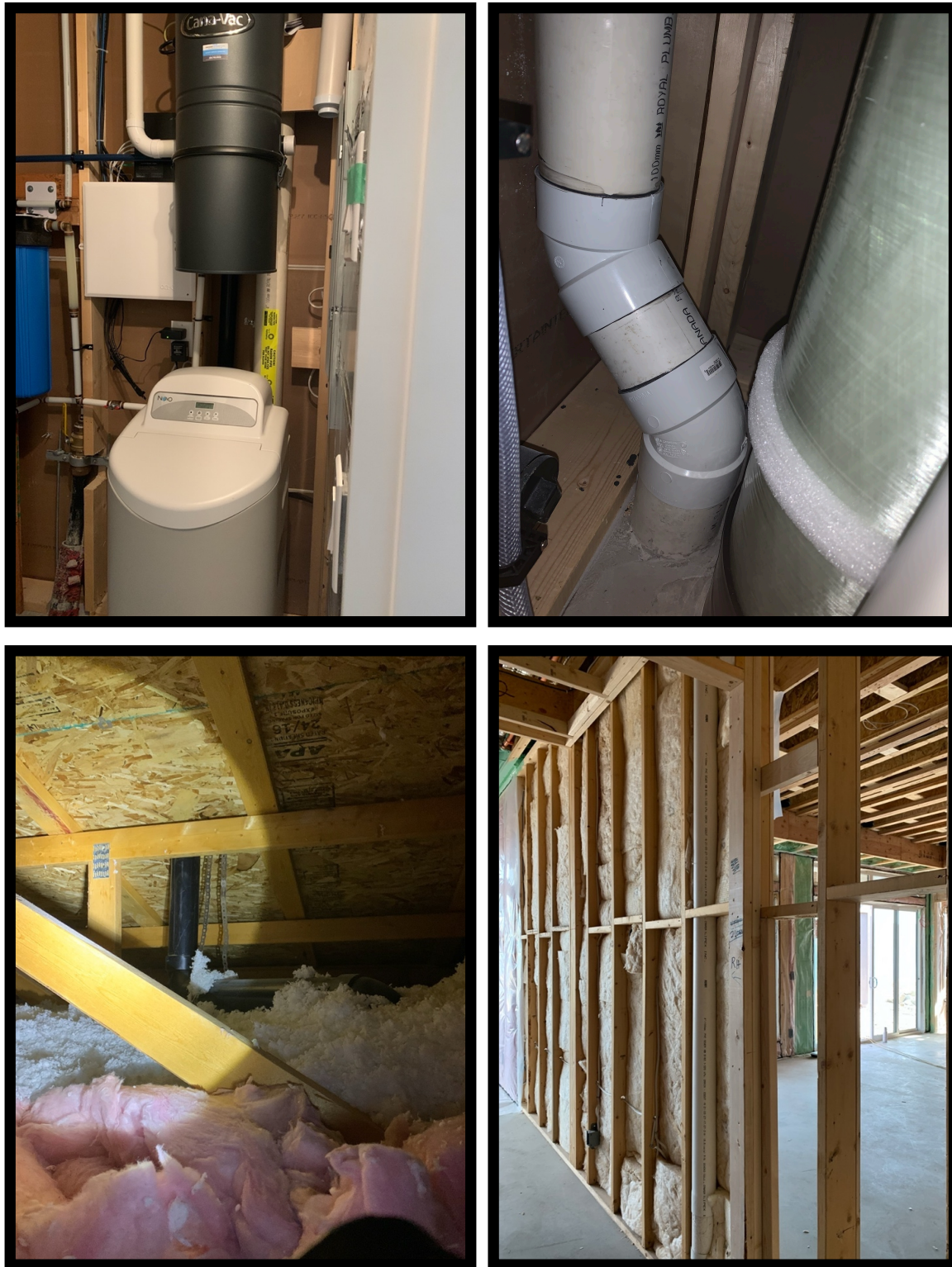
Figure 7: Examples of no room for fan. (a) Behind water heater and central vacuum (top left), (b) behind furnace (top right), (c) squeezed into narrow attic space (bottom left), (d) built into wall assembly, (bottom right). Photos from Chantal Wilson from site visits for this study.
