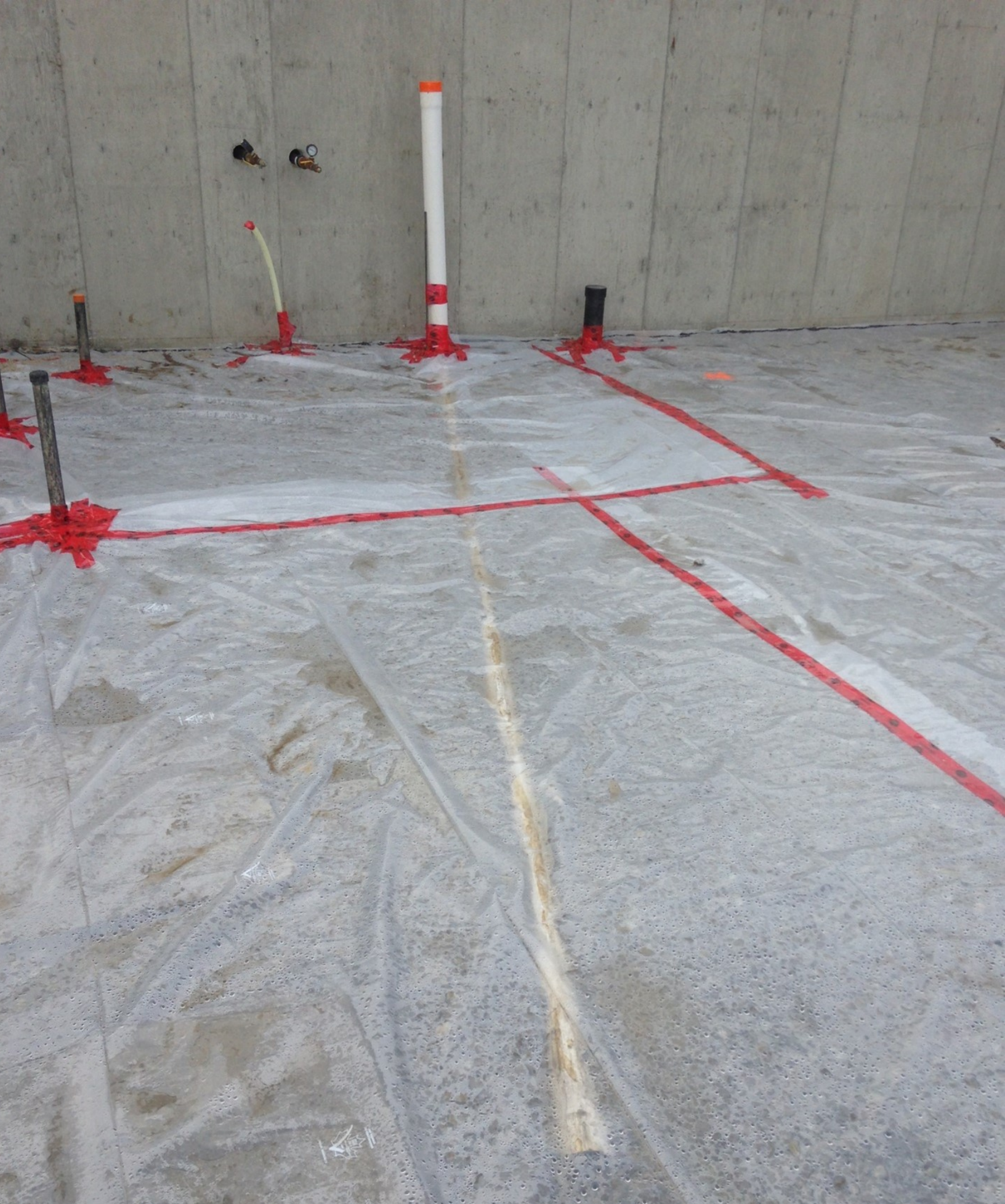
Figure 3: Awkward Soil Gas Collector. Photo credit: John Kostelnick, Okanagan Radon
